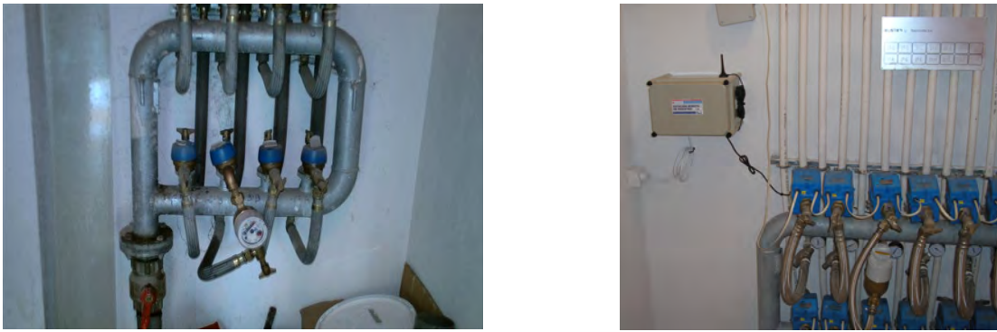
FIGURE 83. METER FOR CONTROLLING WATER CONSUMPTION IN THE HOUSEHOLD (LEFT) REMOTE STATION FOR DATA RECORDING AND TRANSMISSION (RIGHT OF THE FIGURE)
